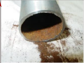
Corroding the inner wall of pipelines
